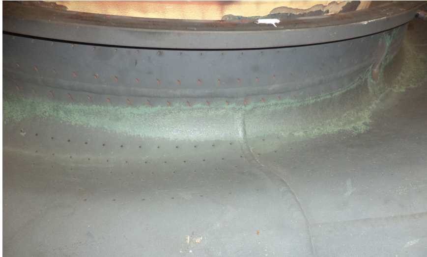
Fig. 44 Green nickel oxide found on the external surface of the analyzed object after service.
